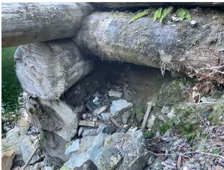
Loosing fill at upstream right bank
