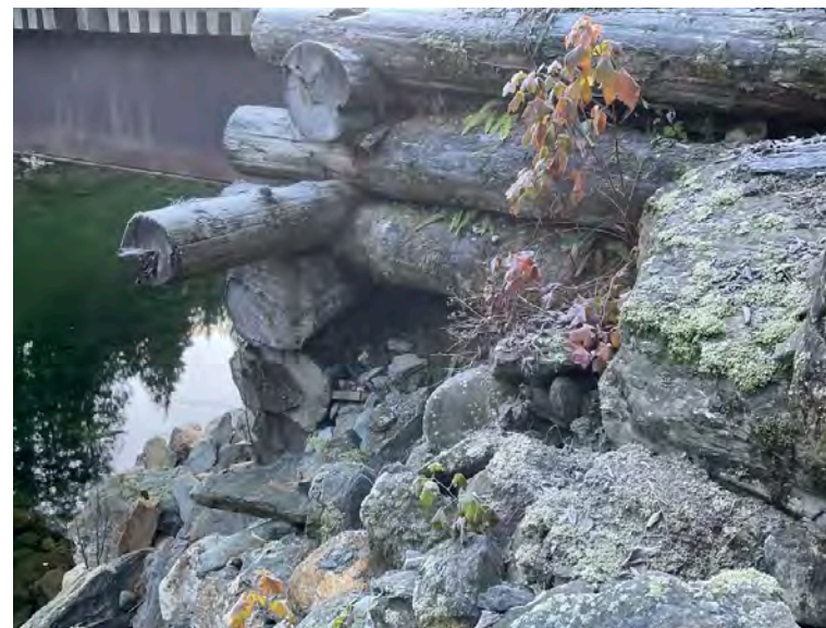
Loosing fill at upstream right bank
