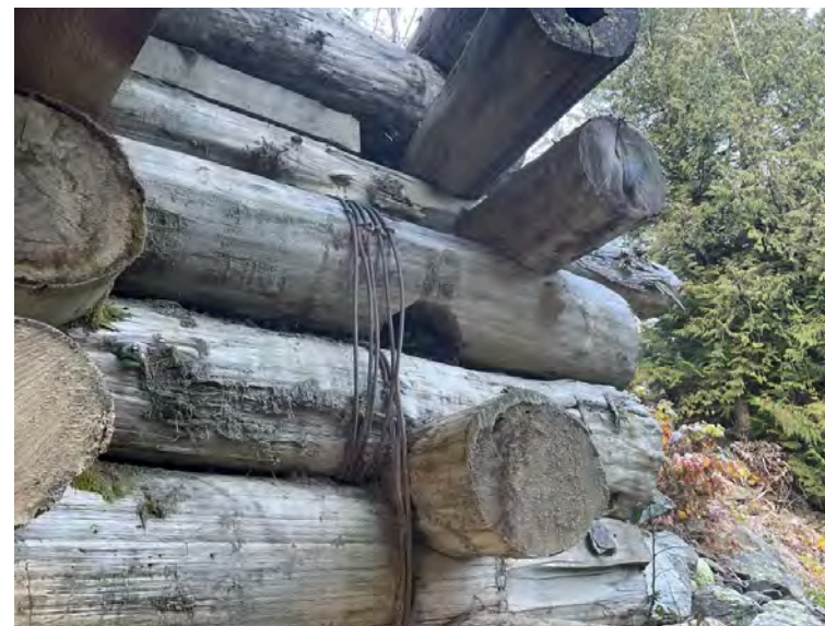
Right bank tieback end missing
