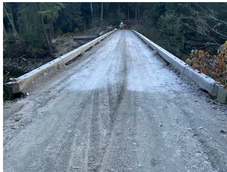
Sediment on deck
