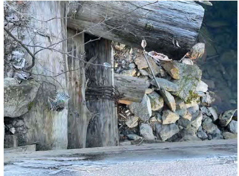
Missing tieback end
