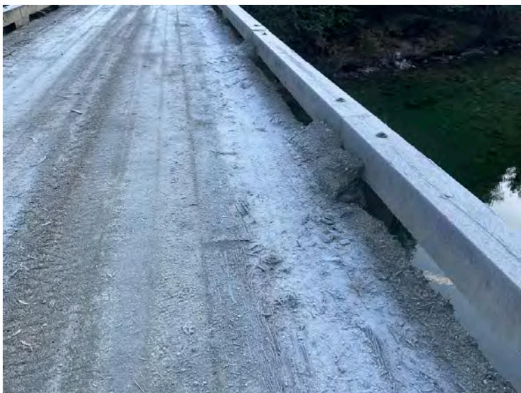
Sediment on deck
